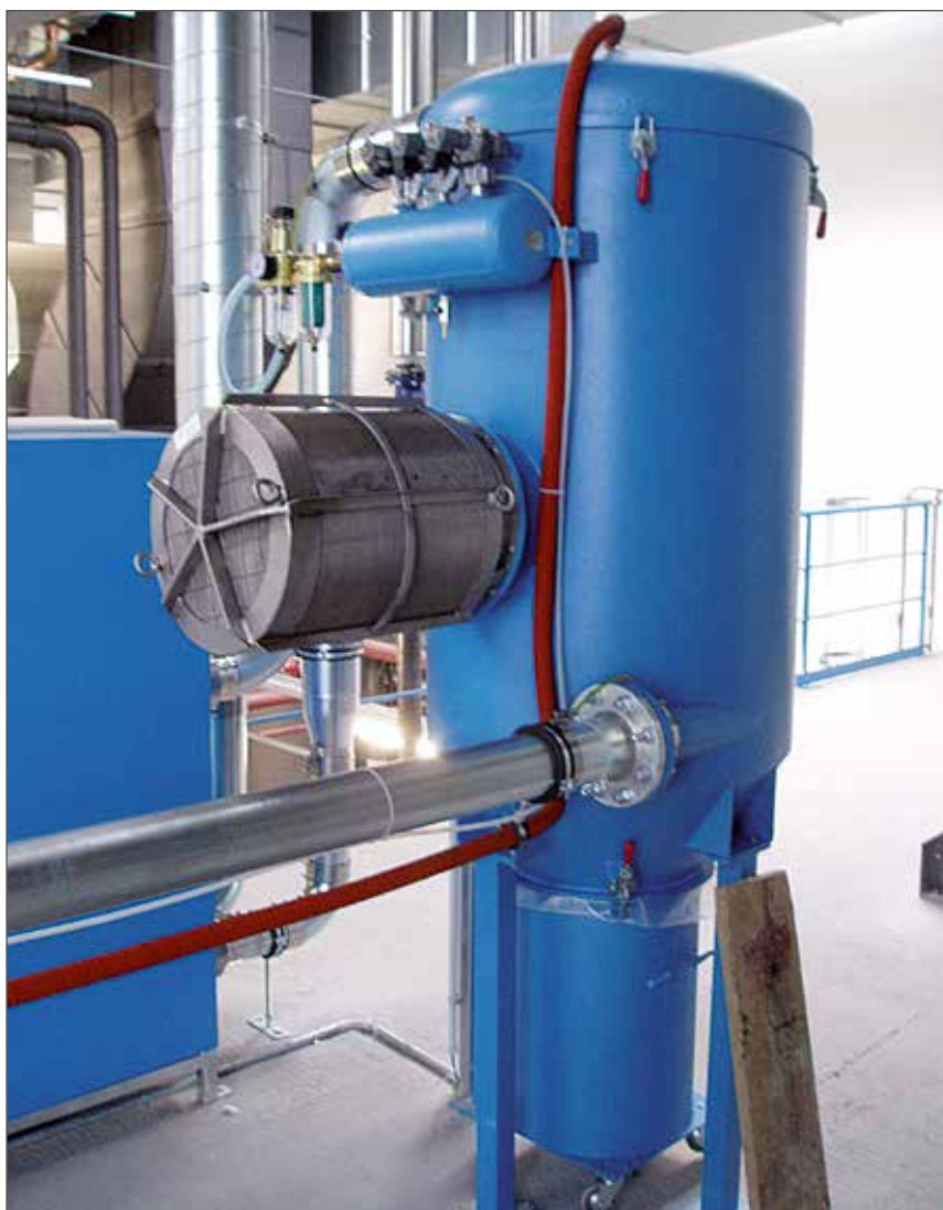
The Q-Rohr protects the suction system at an aircraft manufacturer.
