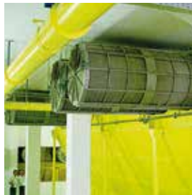
Explosion protection at milling hopper in breweries
