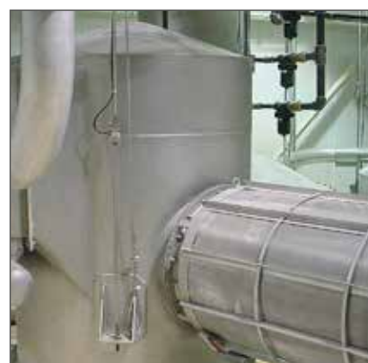
Q-Rohr installed in a recycling plant
