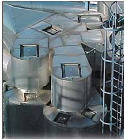
Wood chip plant protected by ODVs
