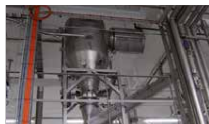
Q-Rohr protects a plant producing grain products
